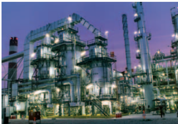
Refinery: Competitive advantages in the project management by accurate planning. (Source: OMV)
